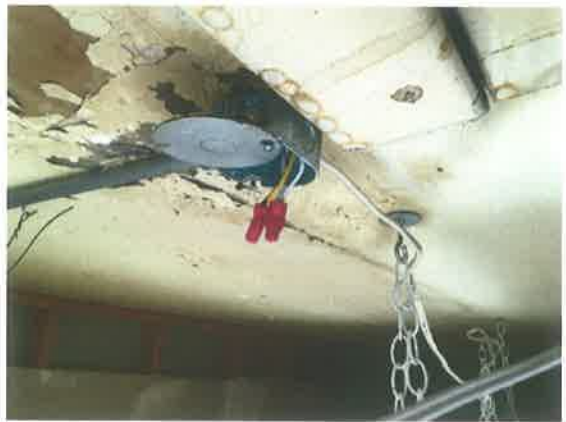
Miscellaneous – Exposed Electrical Wiring
