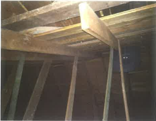
Figure 2: Roof framing as seen from the attic access hatch at the second floor ceiling.
