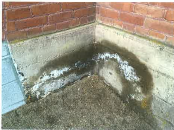
Figure 4: Area of water infiltration in the basement below.
