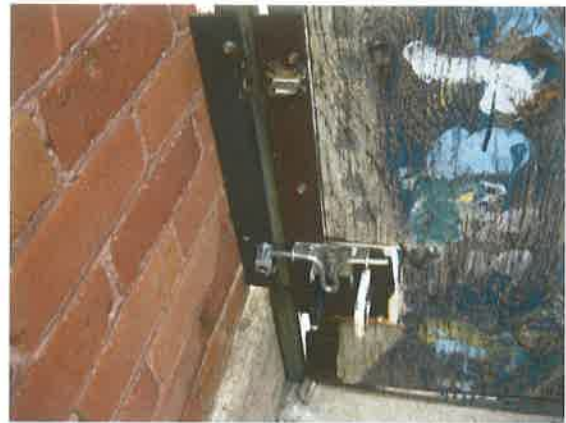
Fire Escape – Gate Bolt
