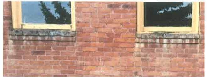
Figure 5: Brick at window sills has deteriorated.
